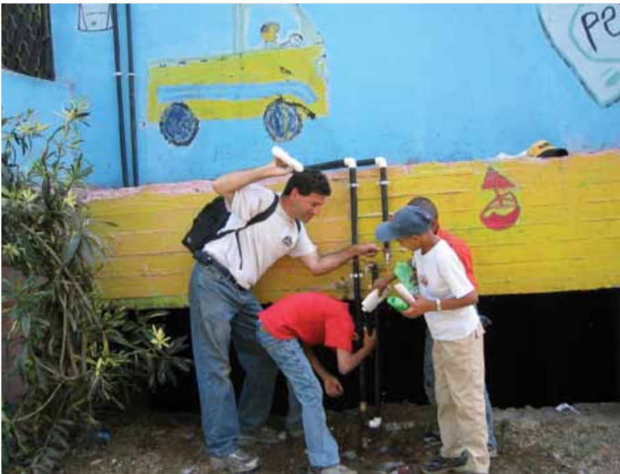
TOP: T. H. on the roof of the Zabaleen Recycling School with Sulaiman (far left), and Milad (middle) after they built their first “hand-made” solar hot water system out of local materials. The water tanks are recycled plastic shampoo barrels, the stand is made out of local bricks brought by donkey cart and the panels absorber plates (under the glass) are made out of recycled butter tins that Sulaiman and Milad cleaned, straightened and painted.
